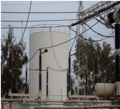
Figure (8) fixed spray washing system in Tripoli east 220 kV S/S
