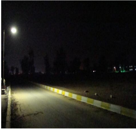
FIGURE (18) PHOTOGRAPH OF THE HIGH POWER LED LAMP WITH LENS MOUNTED IN THE FIXTURE ON THE POLE DURING THE NIGHT
